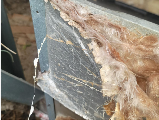
3104-13 Insulation/Wrap Exterior HVAC Unit (East)
