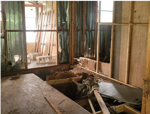
Structural Damage Observed throughout property
